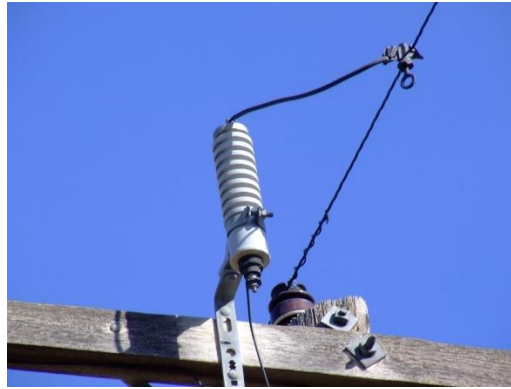
A lightning arrester on a distribution line
